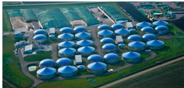
Fermenter, Nachgärer und Gärrestlager einer Biogasanlage Digester, secondary digester and end storage of digestate of a biogas plant
